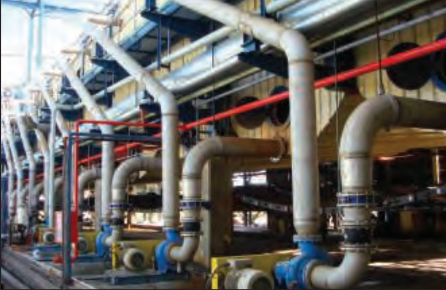
FIGURE 2. This photo shows a typical piping arrangement for a pumping system
